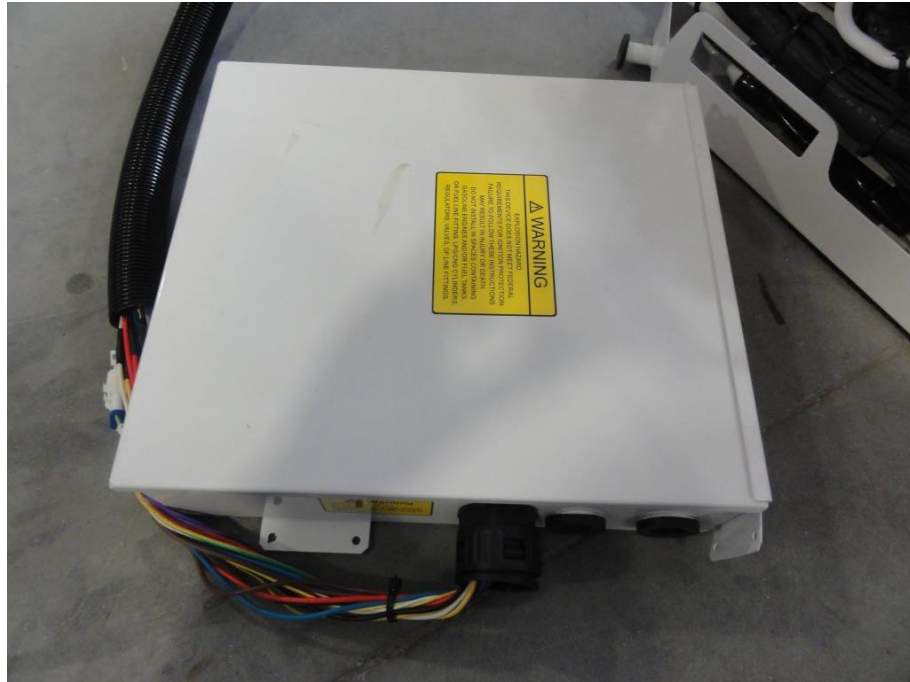
Main power box
